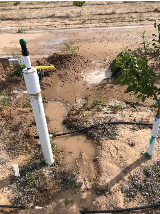
Figure 7. Vandalism (opened valves)
