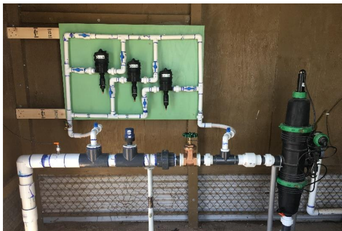
Figure 3. Dosatrons in the pumphouse.
