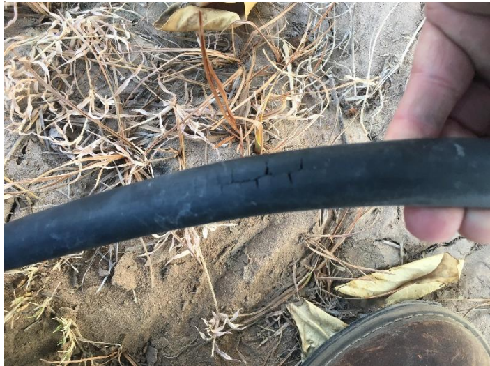
Figure 2. Damage to irrigation line due to UV radiation.
