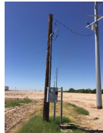
Figure 3. UA Pole and APS High Transmission pole that holds a transformer on the south side of the B Main Lateral canal.
